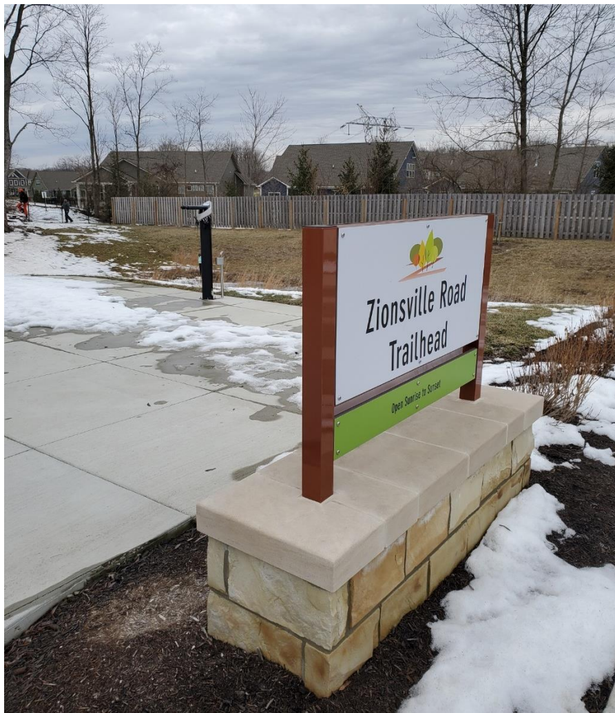
Staff installed a bike repair station at the Zionsville Rd Trailhead as a part of the CIBA grant from 2024. Bicycle safety and trail etiquette signage will join the installation.
