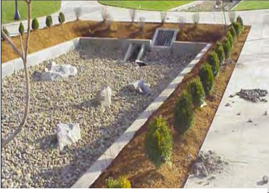
Constructed filter, Portland, OR (City of Portland 2004 Stormwater Management Manual)
