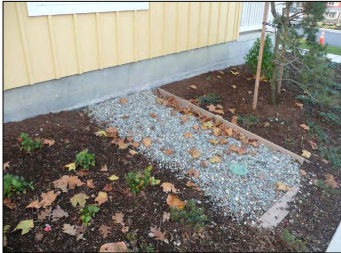
Infiltration bed, Seattle, WA (USEPA, picasaweb)
