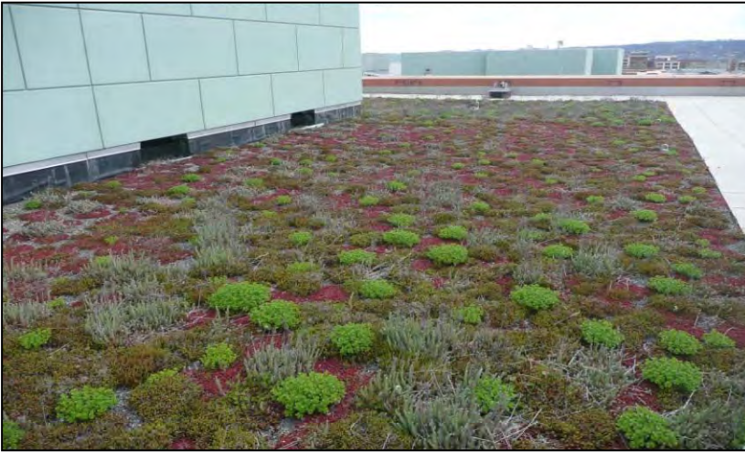
Vegetated Roof, Washington, DC (USEPA, picasaweb)
