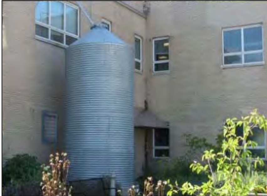
Above ground cistern, Chicago, IL (USEPA, picasaweb)
