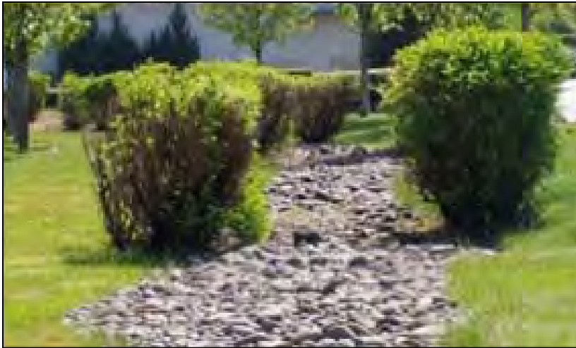
Gravel trench directing water from the parking lot to a vegetated filter strip in Springfield, OR (Springfield Environmental Services Division)
